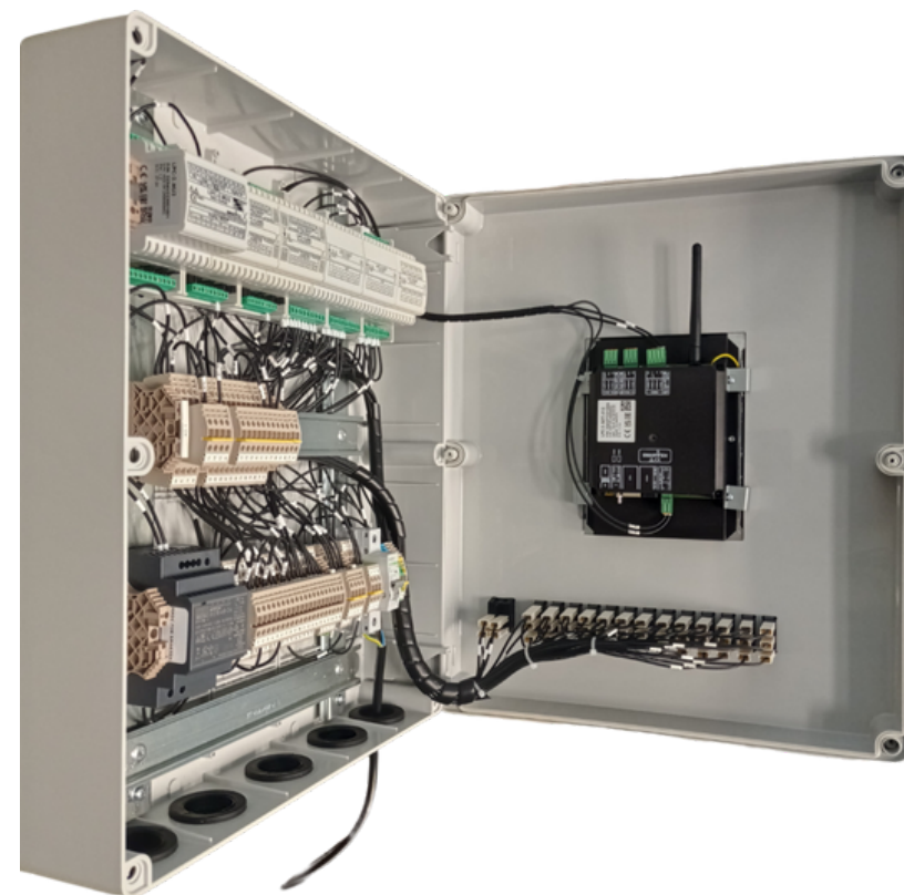
Photo: Interior of the SHC-002 cabinet
